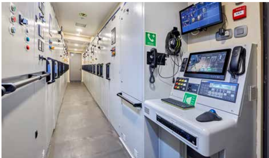
Engine control room for the electric power supply
