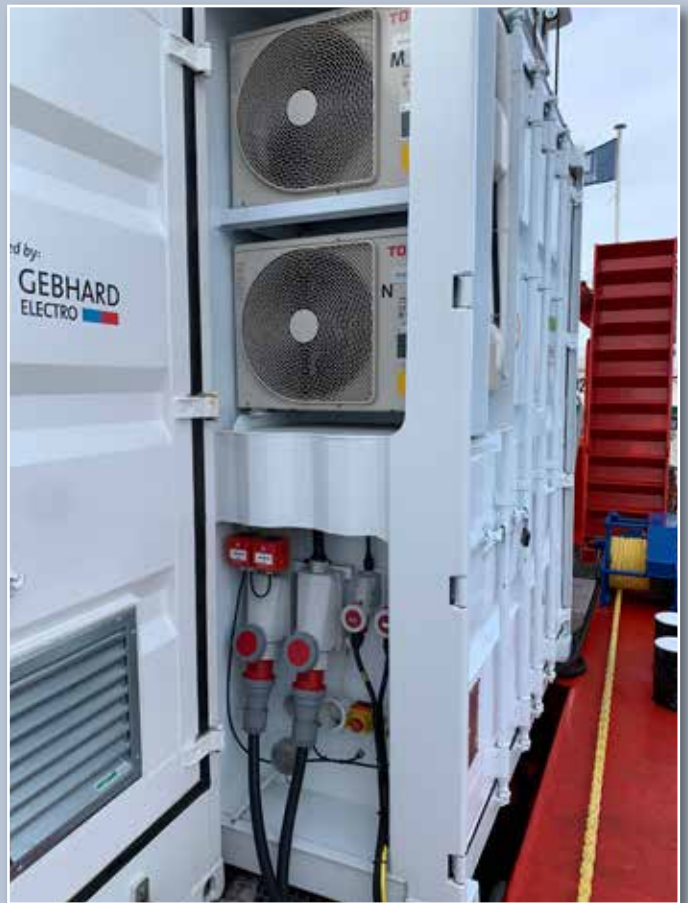
Airco and connectors of the battery room photo: Kotug / Bas van Hoorn
