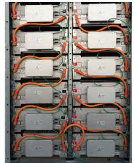
Battery bank photo: EST Floattech
